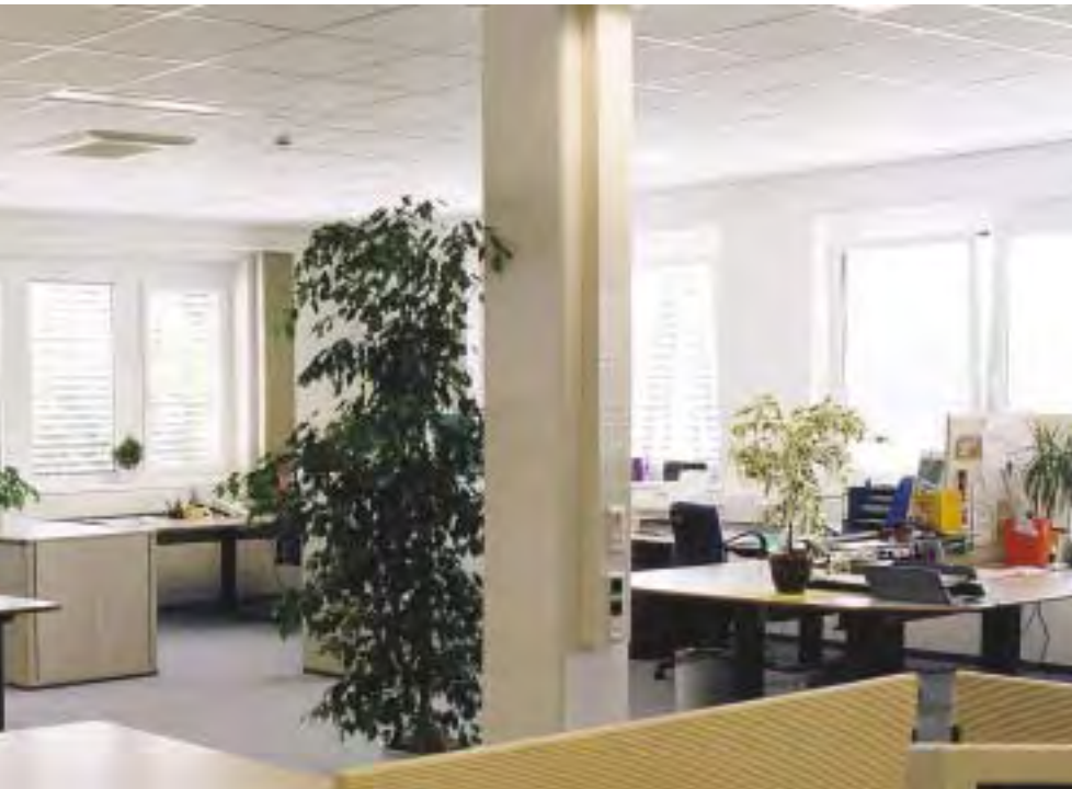
The daylight is measured using an external daylight sensor. Artificial light is added as required.
